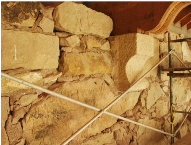
BEFORE: unstable, many openings to the outdoors
