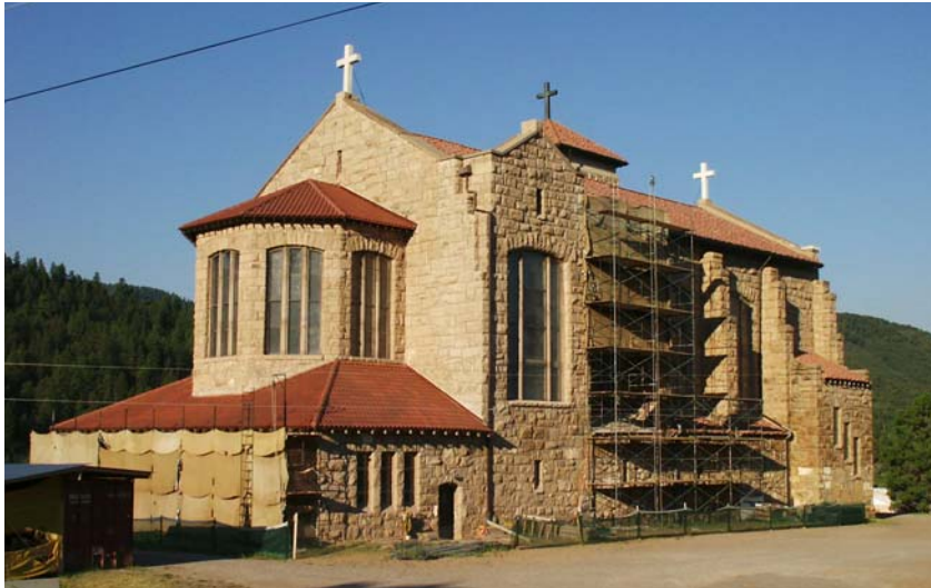
This view shows the two re-roofed sections on the east end of the church, as well as the scaffolding used to complete the repointing on the east end, and the scaffold used to start the restoration of the north wall.
