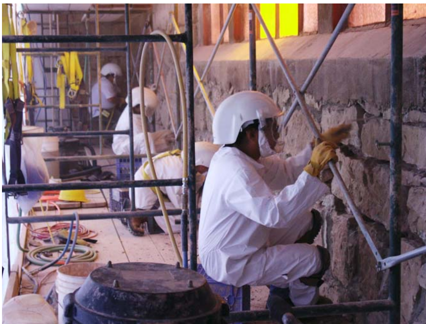
Cleaning out deteriorated mortar – – back to work on the interior of the west wall.
