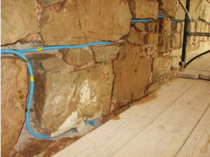
Indoor conduit is embedded in the mortar joints in the west wall interior.
