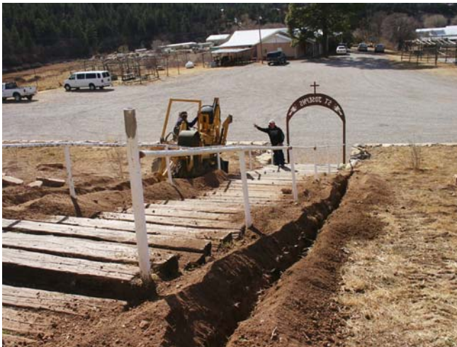
Chris LaPaz of Mescalero Apache Telecom, Inc digging trenches for lights along the steps.
