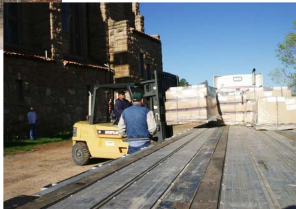
The new clay roof tiles for the east end are delivered to the church, with forklift and operator supplied by the Mescalero Apache Tribe.
