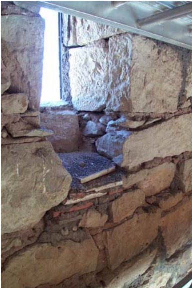
Before: Lower half of window area in bad need of repair.
