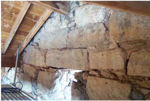
Before: Damage is evident.
