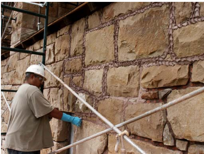
Robert Morgan found some time to do some repointing in between working on the roof. This is the top coat that gets scraped back to get a smooth and finished look.
