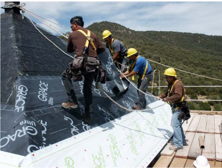
Martin & the roofers, Carlos, Ramon & Mariano putting down the 2 layers of underlayment.
