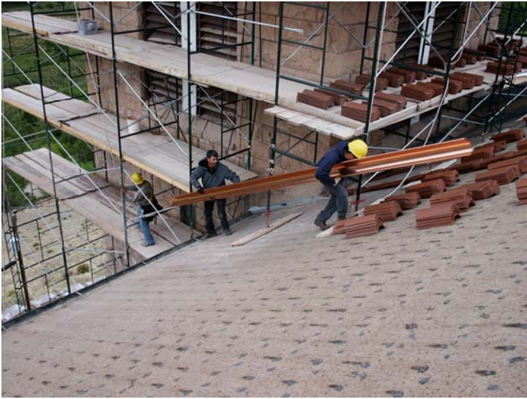
Martin Pizarro and Ramon from McPartlon Roofing Crew carrying up copper gutters for the bell tower roof.
