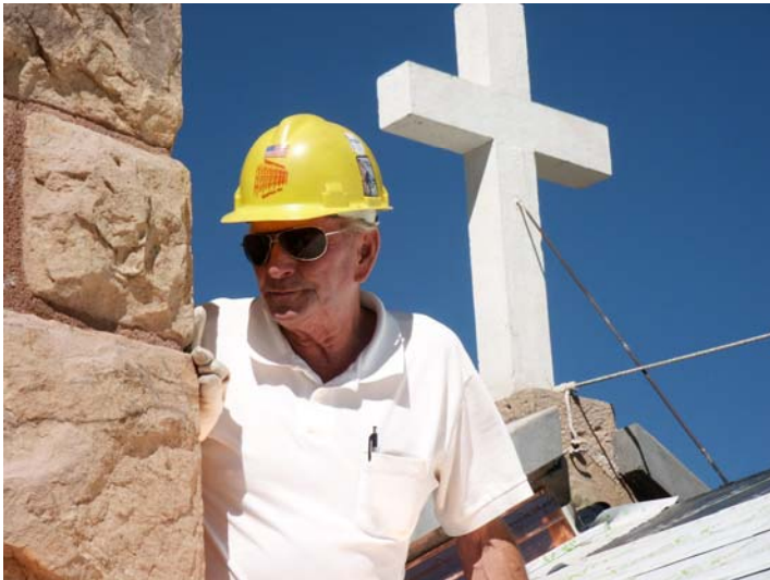
Roy Fleming from Territorial Scaffolding on the roof helping to get the material lift working.
