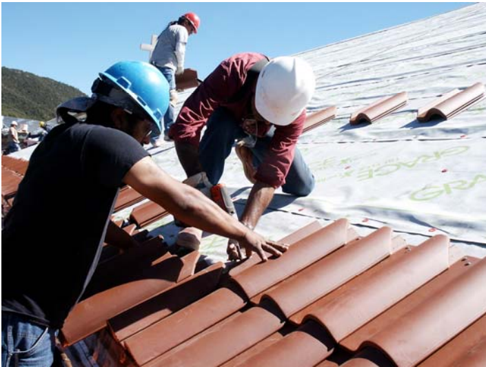
The north side work gets going. Tommy Spottedbird lining up tiles while Sam Sosa helps Andres Ramirez to keep tiles straight.
