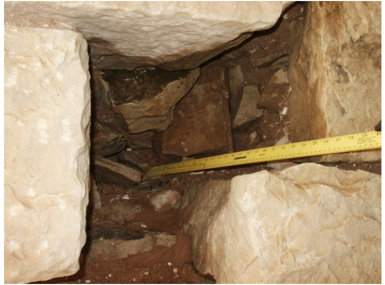
One of the several deep voids.
