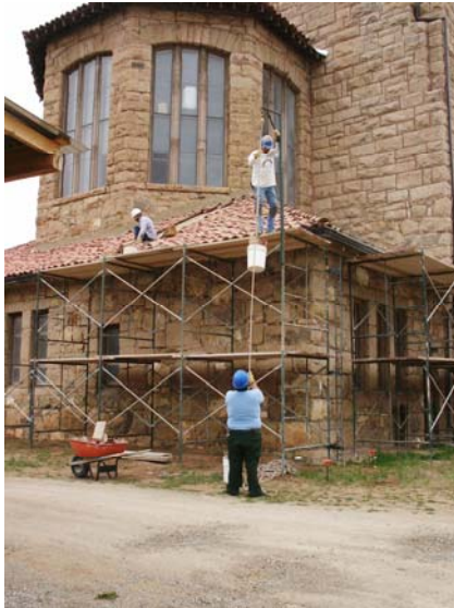
Tommy and Brother Peter removing clay tile while Arylis hoists the tile down in buckets.
